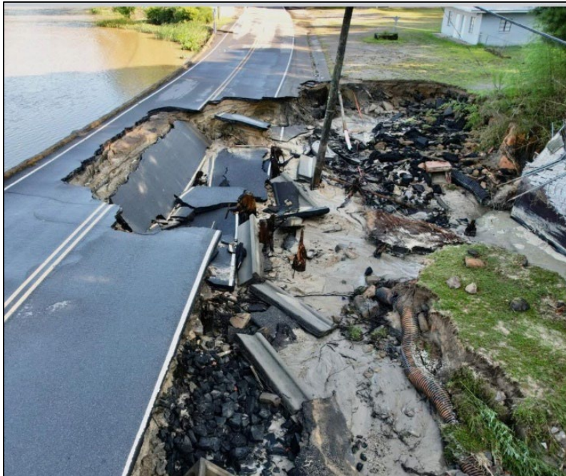
Flooding causes damages to public roads in Moore County. Photo Credit: NCDOT
