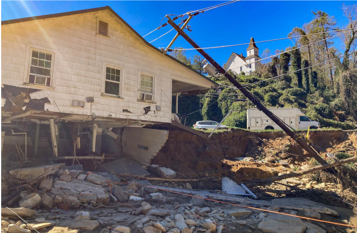
Figure 6: Housing Foundation Damage, US Route 64, Bat Cave, NC. October 10, 2025.
