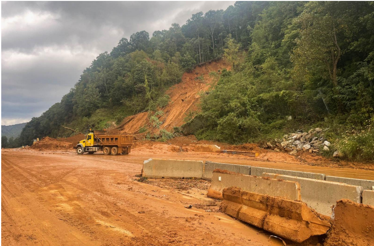
Figure 10: Aftermath of Helene-Triggered Mudslide, September 28, 2024 (Credit: NCDOT)
